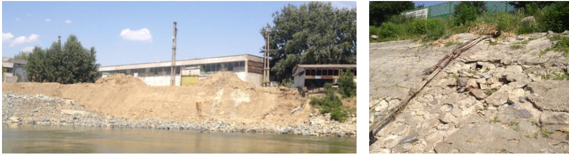
Fig. 1: Area affected by landslide and related damage
